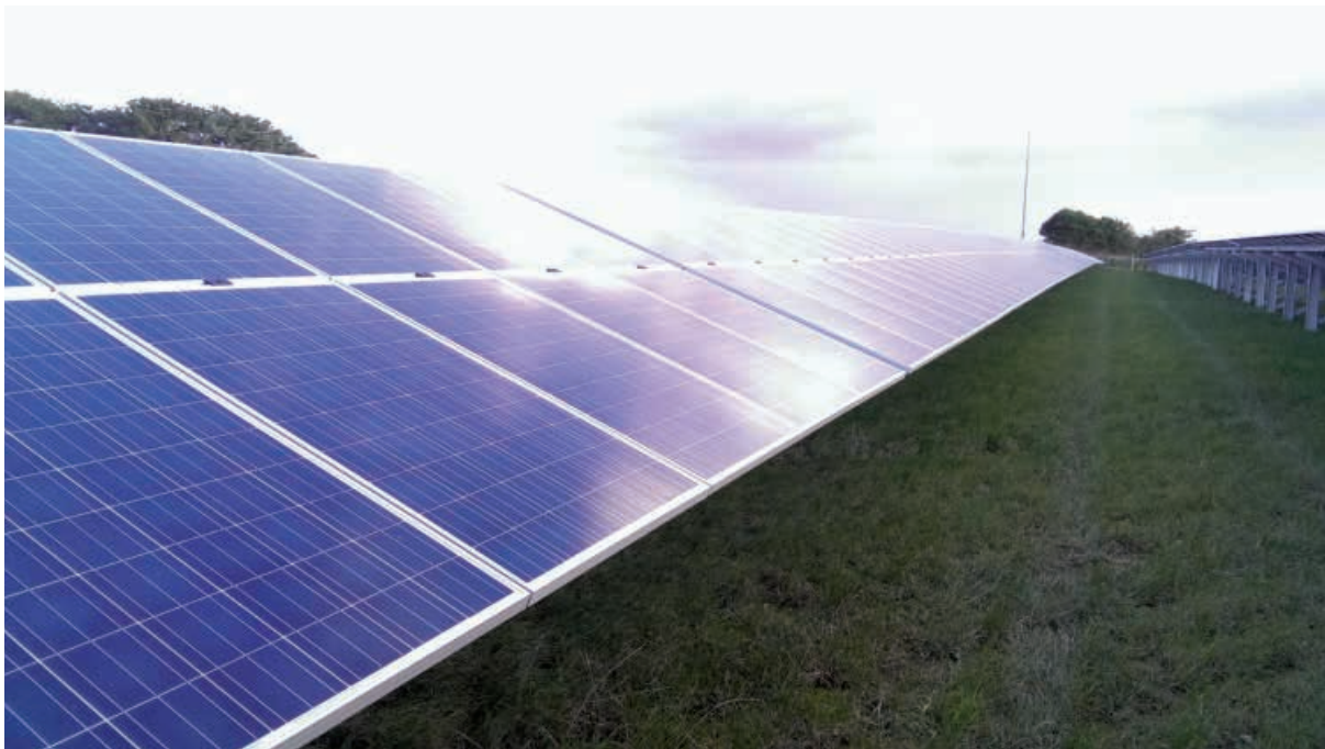
Four Burrows Solar Park, Cornwall, England.
